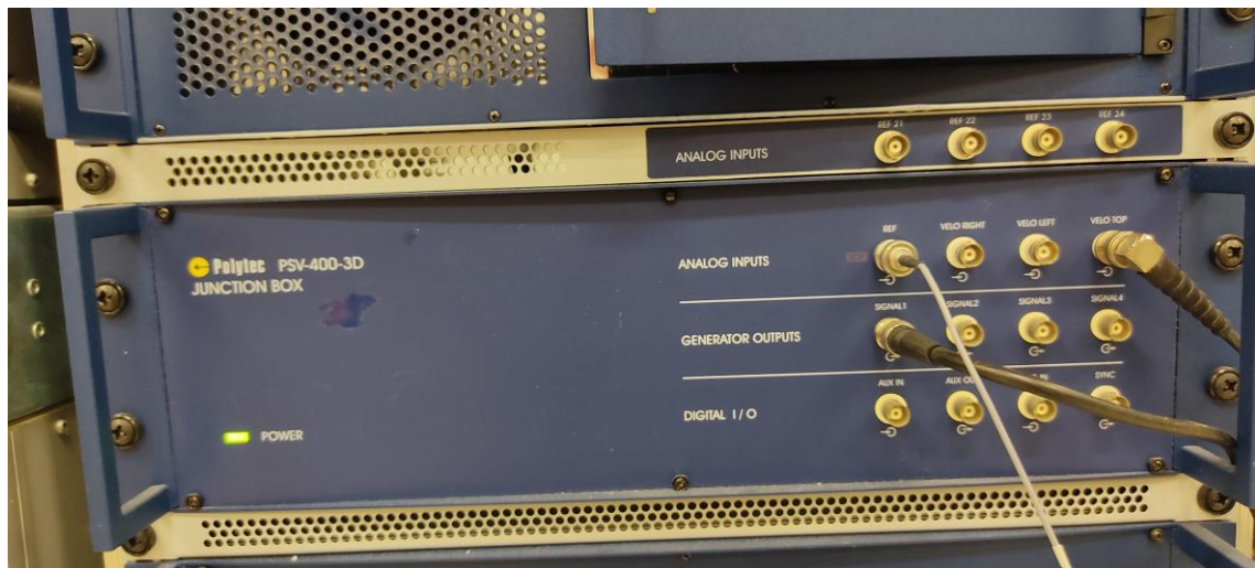
Figura 39 - Detalle cableado Junction Box
